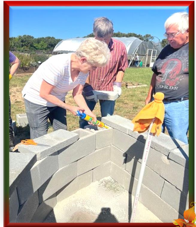
Caps for cinder blocks are being glued down. The white pipe in the foreground is our irrigation line that the Harvest Garden tied into their irrigation system for us.
