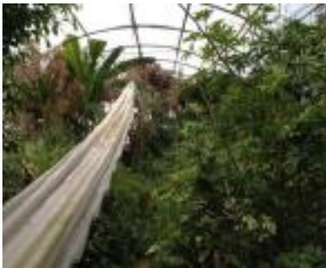
Pictures of greenhouse in disrepair before the partnership with HCMGA
