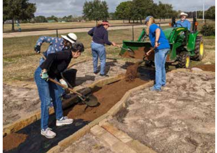
The team filled the walkway with crushed granite delivered by John Ely.
