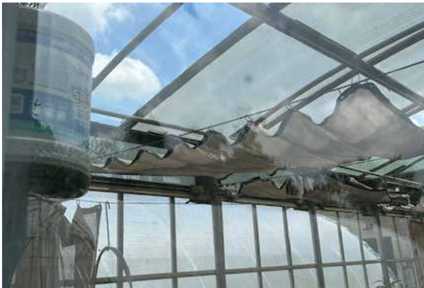
The roof was pulled off the greenhouse.
