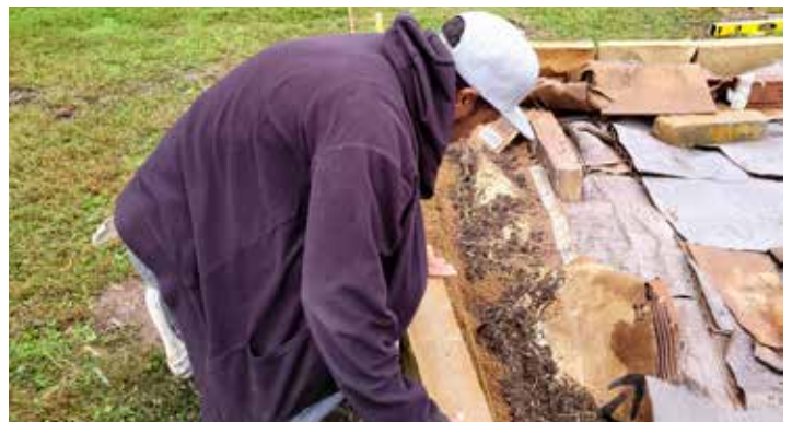
Crushed granite was added to the etched border. Here, Nemo Jackson is leveling an edging stone using the string as a guide.
