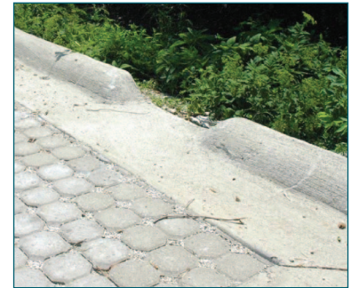
Figure 4. Curb cut opening. (Source: USDA, NRCS)
