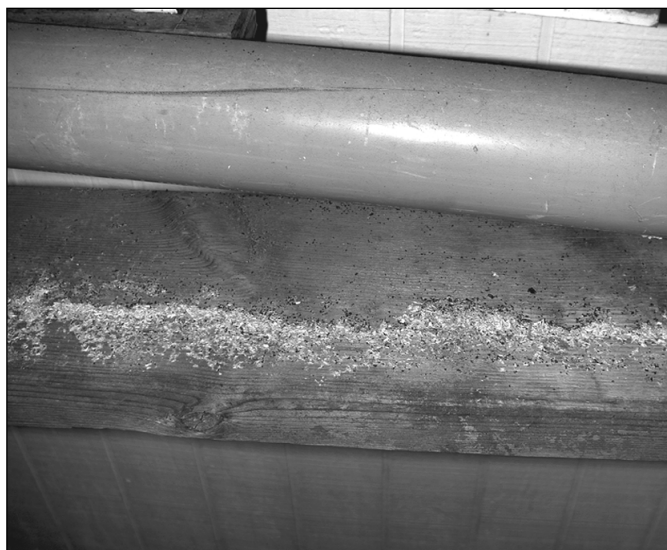
Sawdust accumulation below carpenter bee entry hole.
