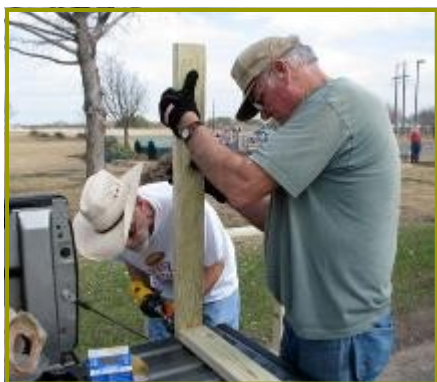
Mike Harper and Chuck McKelley are building a three-bin turning compost unit.
