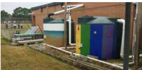
Irrigation and solar panels. All photos MG Don Hogarth
